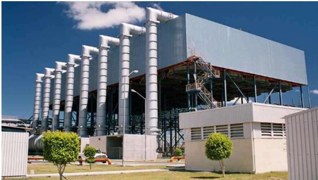
Figure 1.6 Elevated air-cooled condenser array (SPX, 2015)
